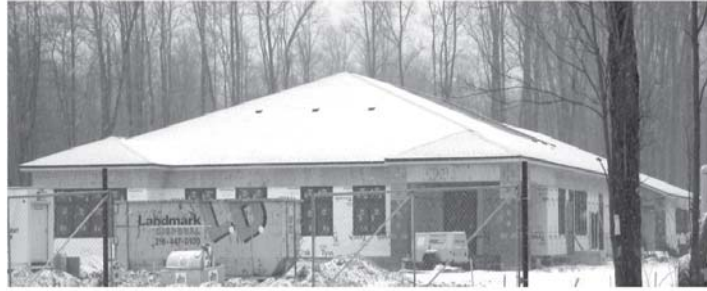
The Green House is scheduled to open this summer! A roof, windows and electric were only a portion of the completed projects in the 26th week of construction.
